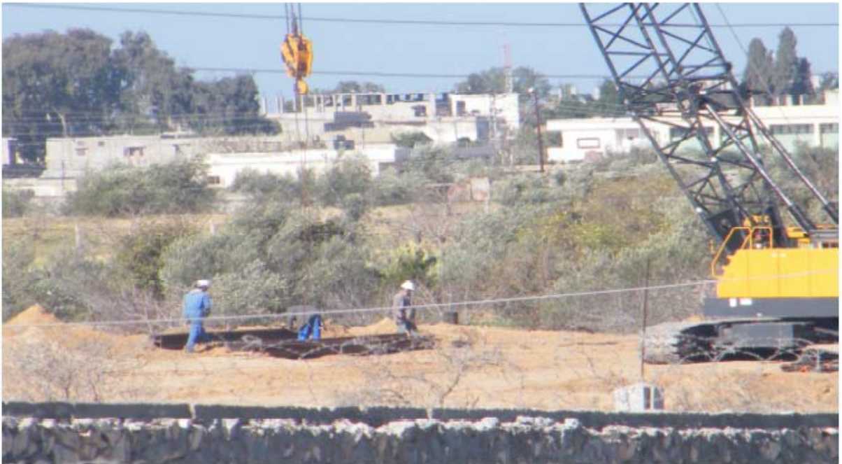
A set of photos taken during the process of drilling for the construction of the steel wall on the border with the Gaza Strip
